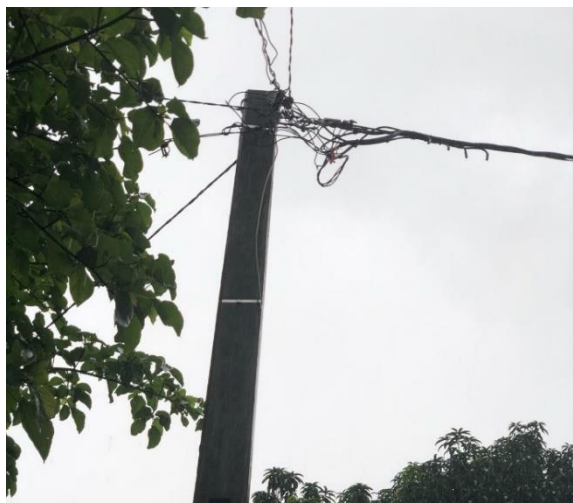
Due to poor infrastructure, the inhabitants of the capital Conakry suffer from regular power outages.
