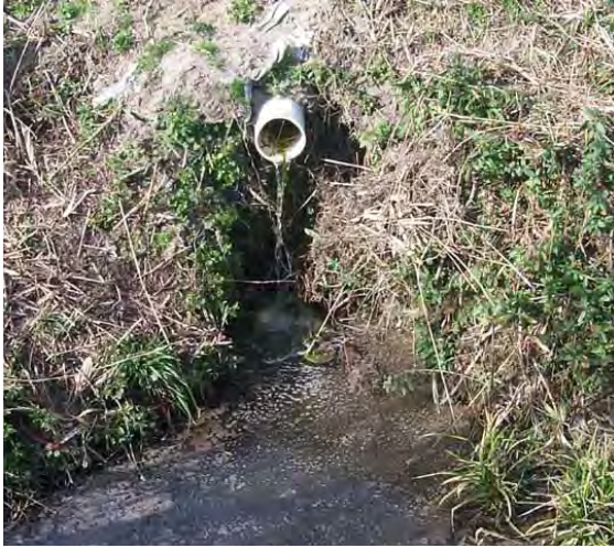
Tile drainage lines run under the surface of agricultural lands and channel water off the farm, sometimes causing erosion and depositing nutrients and chemicals at the end of the line. USGS photo.
