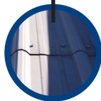
open or lifted seams
