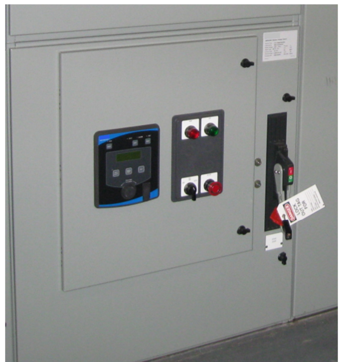
Fig. 10: Each starter cubicle includes a starter display module (SDM). Door mounted discrete control devices were included for ease of interface to the existing DCS
