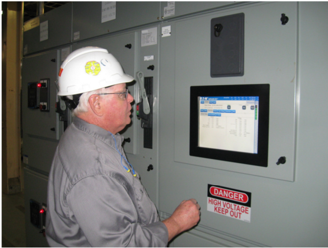
Fig. 8: Mill engineer stands in front of Central Display Module of the new motor control center.
