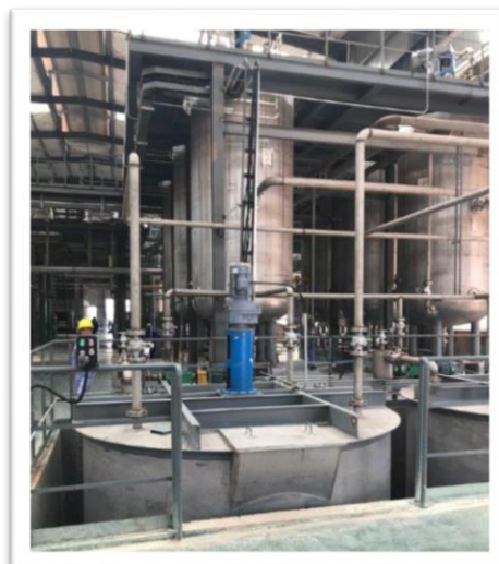
FIGURE 5: BICARBONATION TANKS USED IN THE UPGRADING OF LITHIUM CARBONATE
