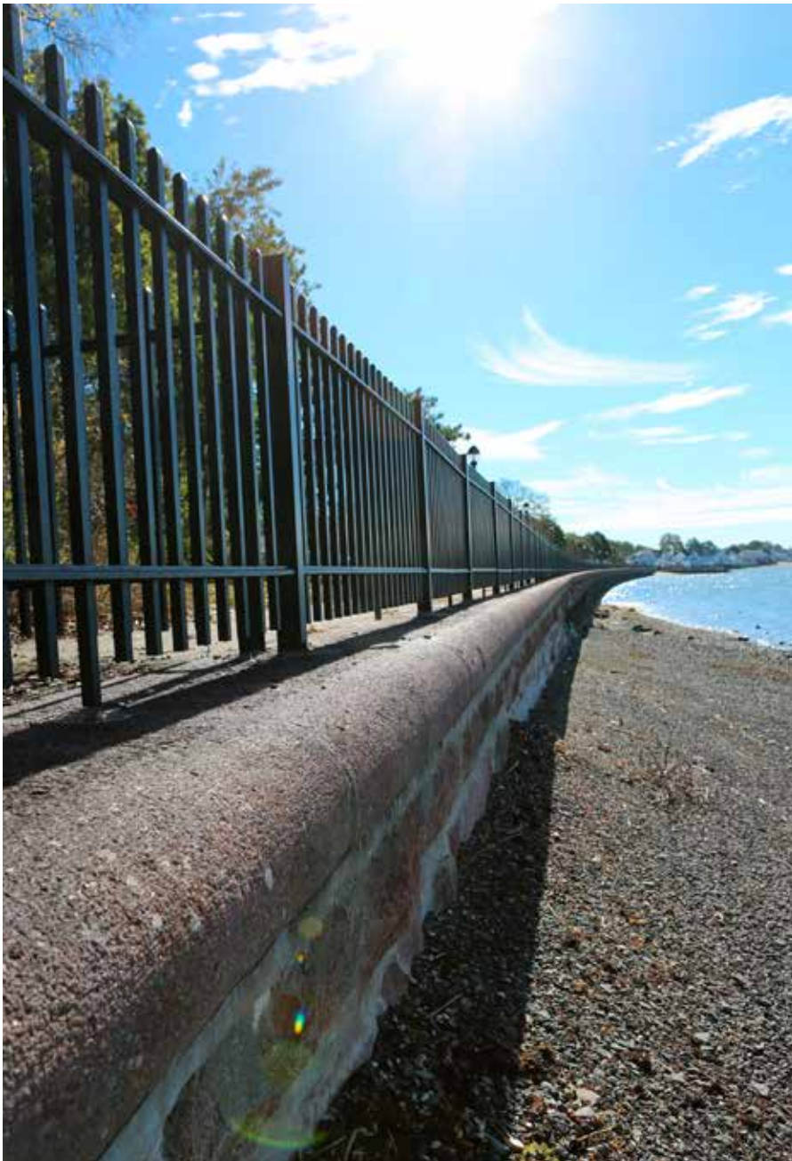
Pardee Seawall. Photo by Todd Fairchild
