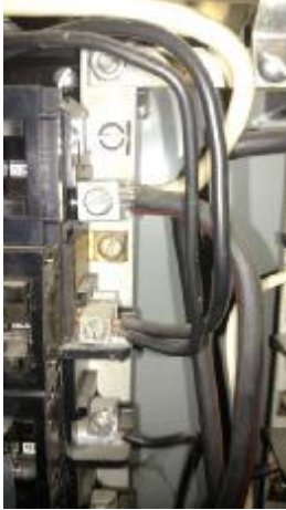
double tap breakers
