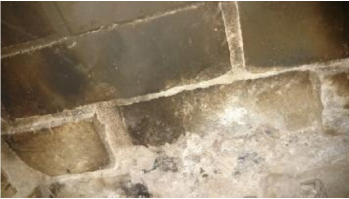
Damaged fire brick
