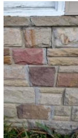
Crack in veneer
