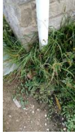
Poorly located down spout
