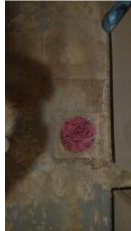
No drain screen
