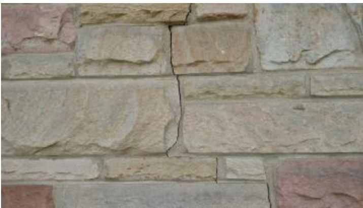
Crack in sandstone veneer
