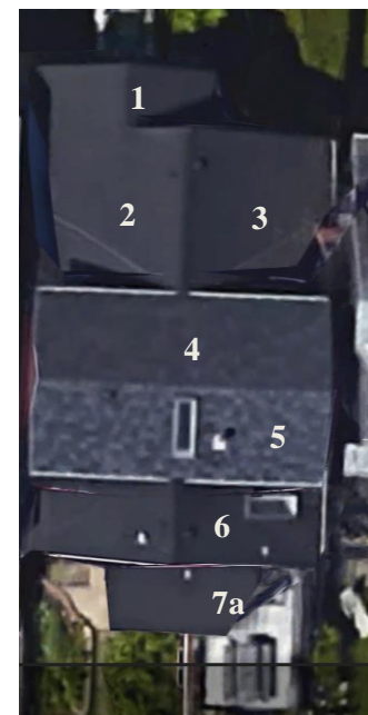
Figure 2: Existing Assemblies Area 1, 2, 3 & 6: Unvented Vaulted Ceilings Area 4 & 5 : 2006 Dormer Extension: Area 7:- Open to below – no insulation Page 1 of 6
