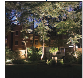
Garden lighting installed at Hill-Physick and Powel House
