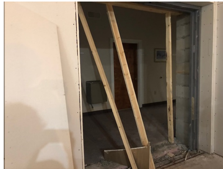
Doorway from existing upstairs Sunday School classrooms to second level in new sanctuary
