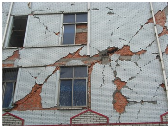
Fig. 1 Damage of RC building with masonry infill in China 2008 Wenchuan earthquake
