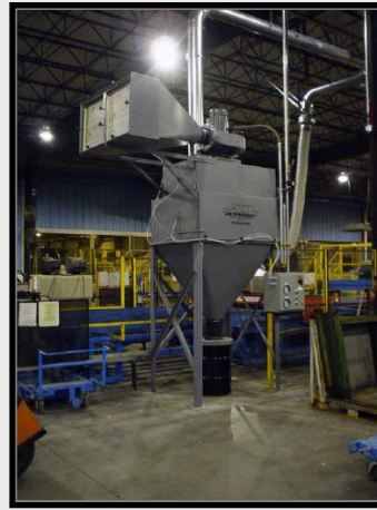
Dust Collection Unit
