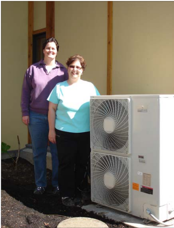
Bauman and Broussard ended up with the first installation of the Daikin Altherma™ system in the U.S. - a tremendously eco-friendly heating and hot water supply solution.
