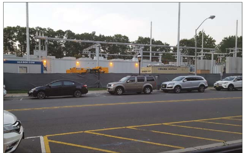
REBUILDING SUBSTATION... The PSE&G substation in Cranford is in the process of being rebuilt. It is seen on Saturday from the outside patio of the River & Rail restaurant across the street.
