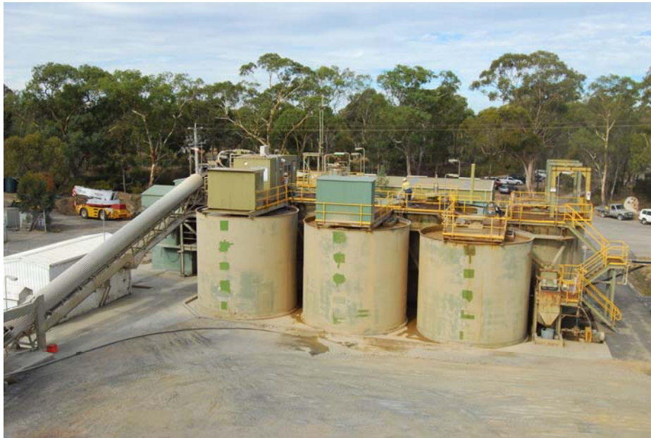
Figure 1. Operating Maldon Treatment Plant Monday 2 nd March 2015
