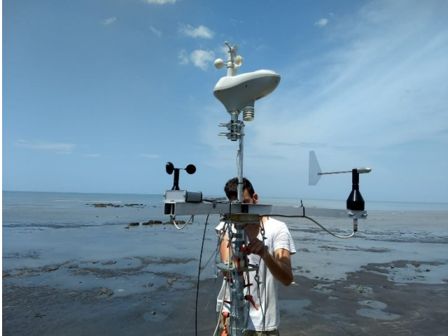
Installation of the measuring system developed by SINN Power.
