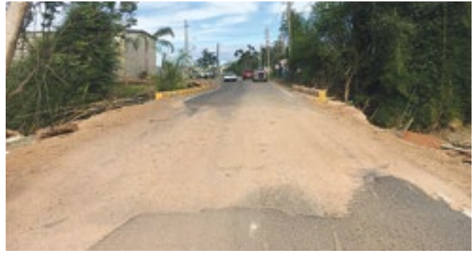
Fig. 9. Damage at approach pavement on Bridge No. 256, San Sebastian PR
