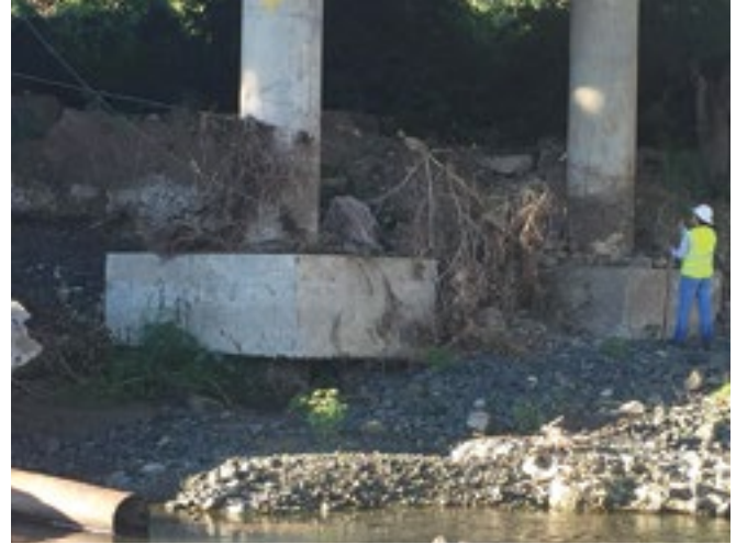
Fig. 6. Scour and exposed footing and piles at interior pier of Bridge No. 2086, Sabana Grande PR
