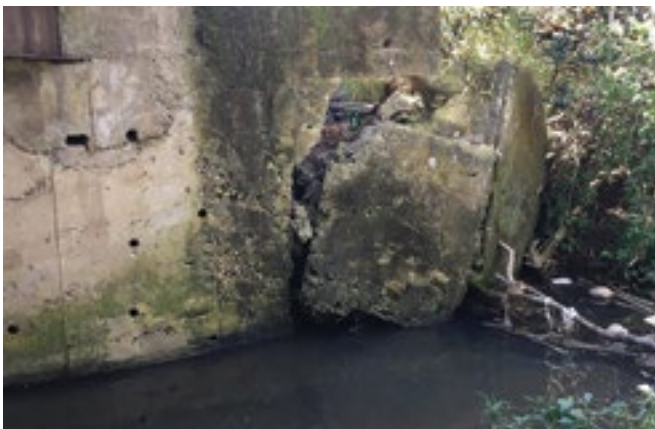
Fig. 4. Upstream partial wingwall collapsed Bridge No. 141, Cabo Rojo, PR
