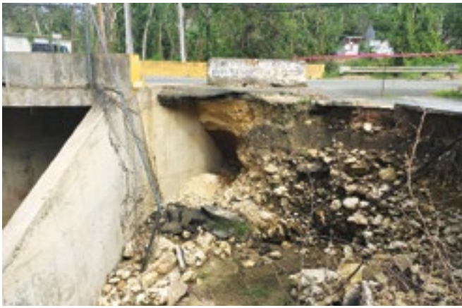
Fig. 3. Downstream wingwall slope instability Bridge No. 446, San Sebastián P.R.
