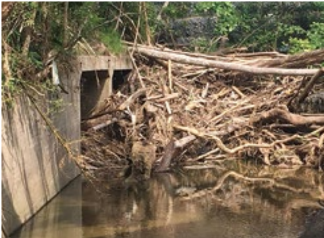
Fig. 8. Typical debris at low elevation multi-cell box culvert type bridges.
