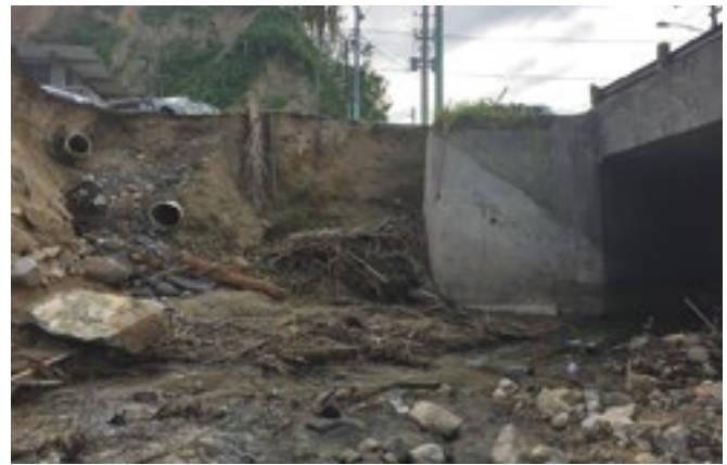
Fig. 2. Upstream embankment landslide Bridge No. 879, Utuado PR
