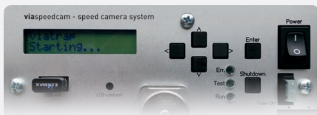
Control panel inside the battery box.
