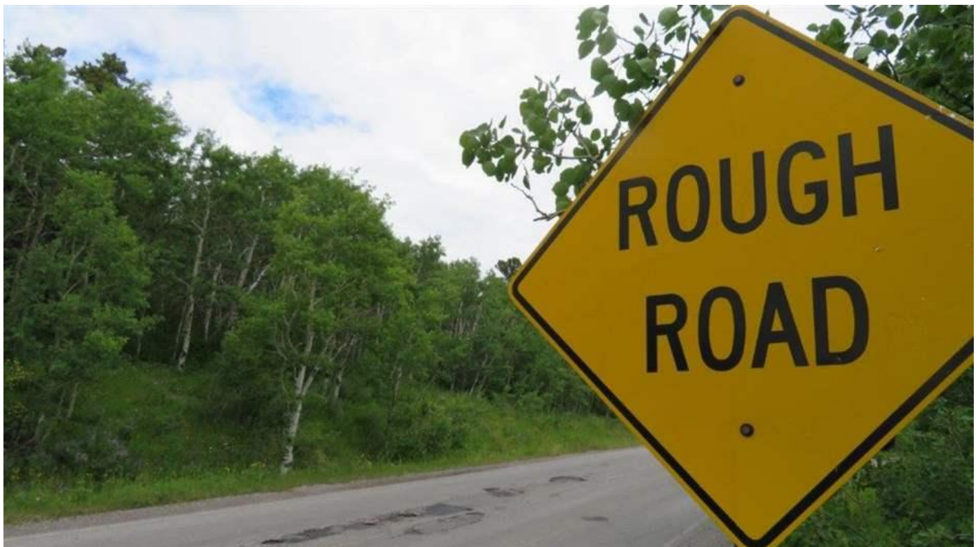
The potholes and cracks on this road in Glacier National Park show how National Park Service assets can degrade when routine maintenance is deferred.
